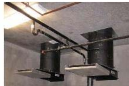
Figure 3: Garbage and recycling chutes
